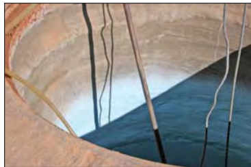
The bright, highly reflective blue epoxy coating nears the top of a manhole.
